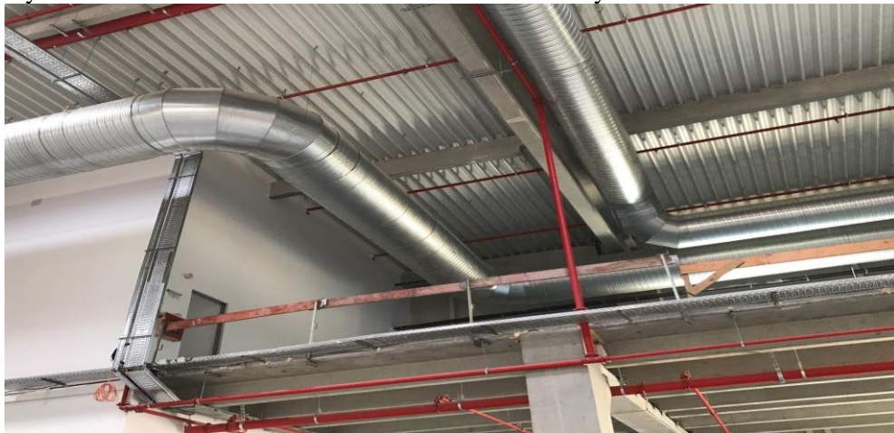
Fig. 2. The industrial ventilation system
